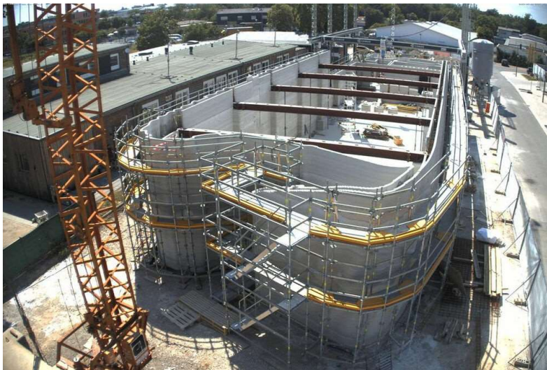
Figure 5: Construction of a Shell for a Data Center Using the 3d Printing Process
